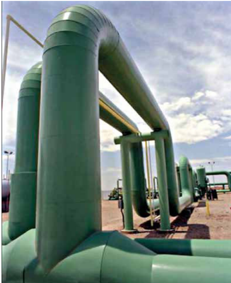
Hydrogen pipelines. Hydrogen is recognized as the foundational element of heavy-industry decarbonization Picture: Wikimedia
