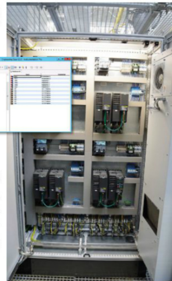
Power range in the cabinet for four booths; project structure in Engineering Base (EB)
