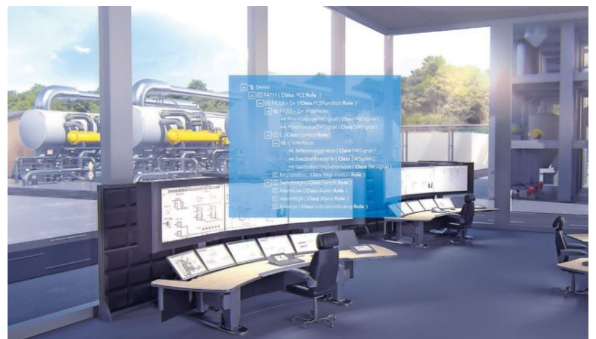
EB also passes on its neutral data to other systems, e.g. control system configuration
